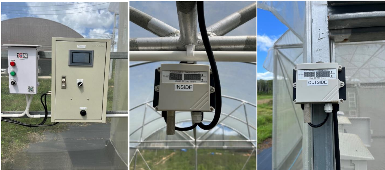
Figure 2 Ventilation control, Temperature and Humidity sensor
