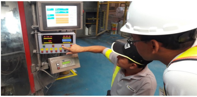
Fig.9. Testing of the data logging control cabinet.
