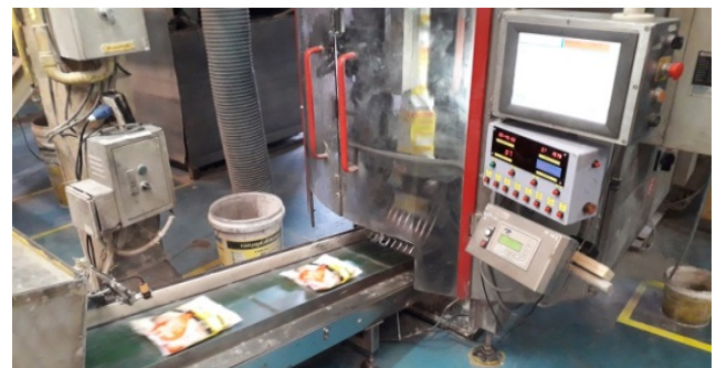
Fig.8. location of the installation of the control cabinet
